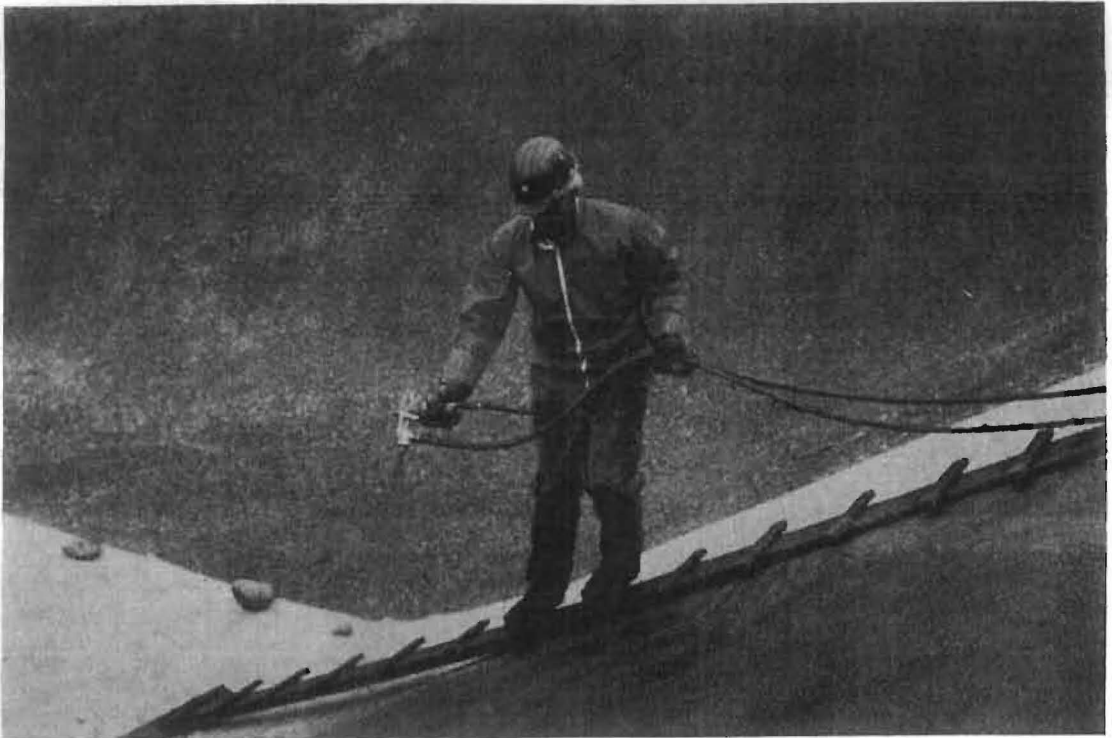
Fig. 4 Wastolan Red is sprayed with air in the low pressure method to penetrate a fleece for tightening a pit.
