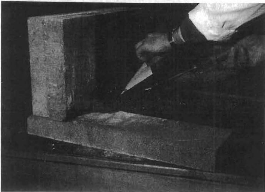
Fig. 2 A fleece being applied to a construction joint precoated with Wastolan. The Wastolan penetrates the fleece giving a reinforced cornice over the joint.
